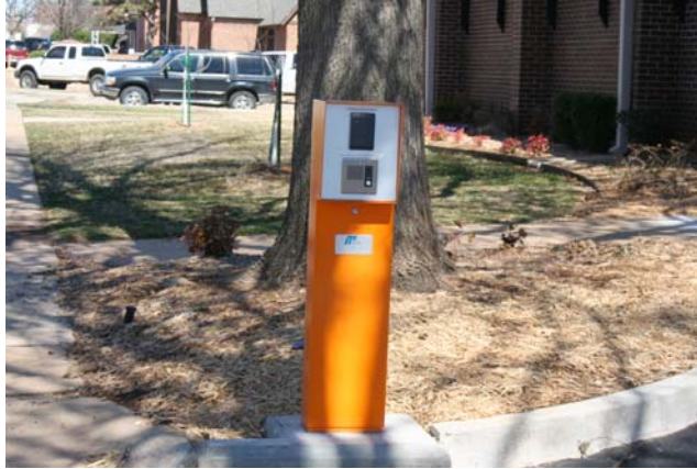
MIDI CONTROL COLUMN WITH PROX CARD READER AND INTERCOM INSTALLED
